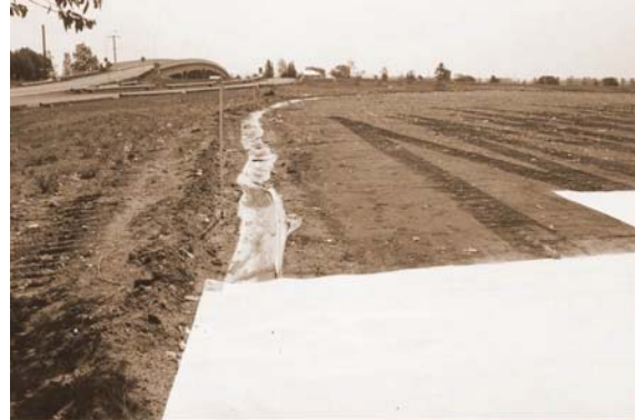
Figure 6: Passive collection trenches beneath the GCL cap.
