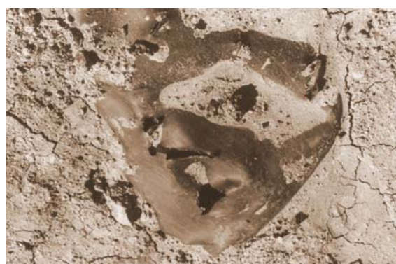
Figure 2. Water tightness maintained after damage to HDPE in a composite liner.
